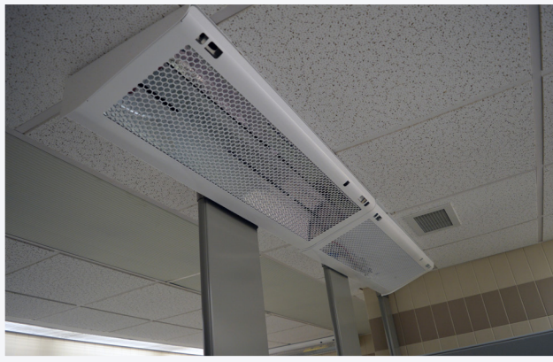
Pictured are two UVC lights in a public washroom by Woodstock Hospital's cafeteria on the lower level of the hospital.
