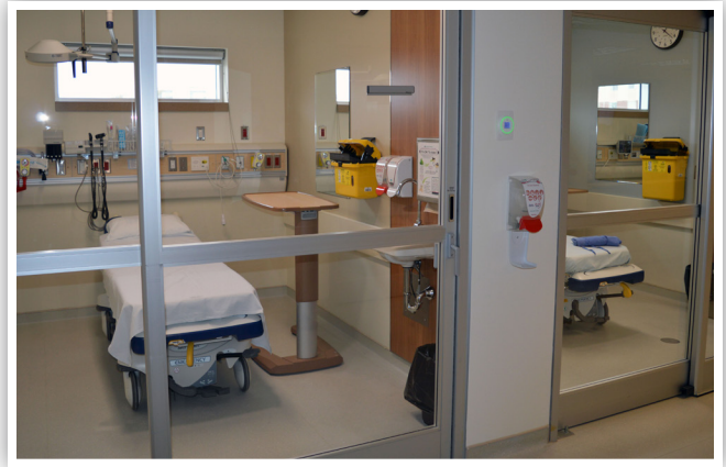
Photo of two negative pressure rooms in the hospital's Emergency Department. The ventilation in these rooms allow no contaminated air to escape them.
